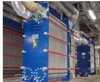
排水・工業用水の排熱回収設備の導入 (2007) Introduction of waste heat recovery system for wastewater and industrial water (2007)
